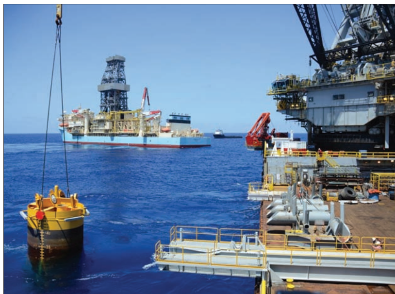
Subsea pile installation at the Julia Phase I project in the Gulf of Mexico.
